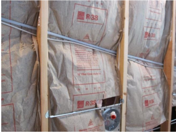
Figure 1 - This faced fiberglass batt insulation was incorrectly installed ; it should be cut to fit around wiring and obstructions so that it can completely fill the wall cavity without compressions and voids
