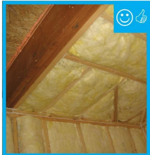
Figure 4 – This unfaced fiberglass insulation has been correctly installed to completely fill the wall cavities and is sliced to fit to eliminate compression of the insulation or voids and gaps in the insulation.
