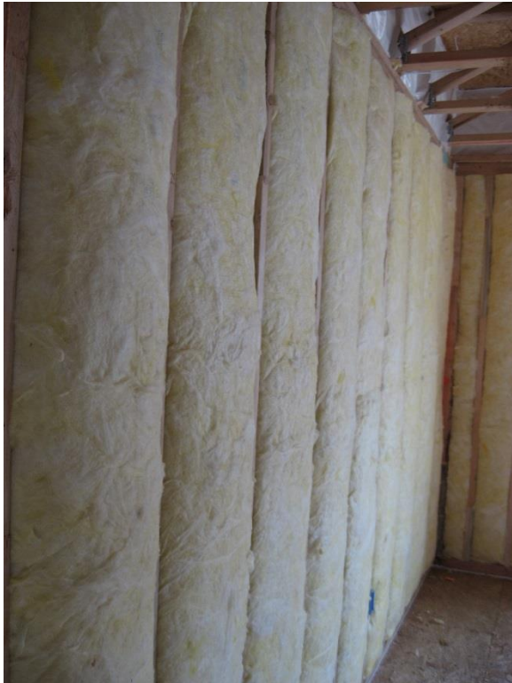
Figure 2 - Unfaced fiberglass batt insulation is correctly installed to completely fill the wall cavities and is sliced to fit around wiring, piping, and other obstructions in the wall cavities without compressing the insulation.
