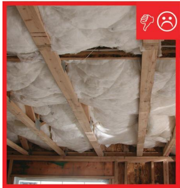
Figure 3 – This unfaced fiberglass insulation has been incorrectly installed due to misalignment, compression, and gaps; it should be cut to fit so that it can completely fill the cavity without any compressions and voids.
